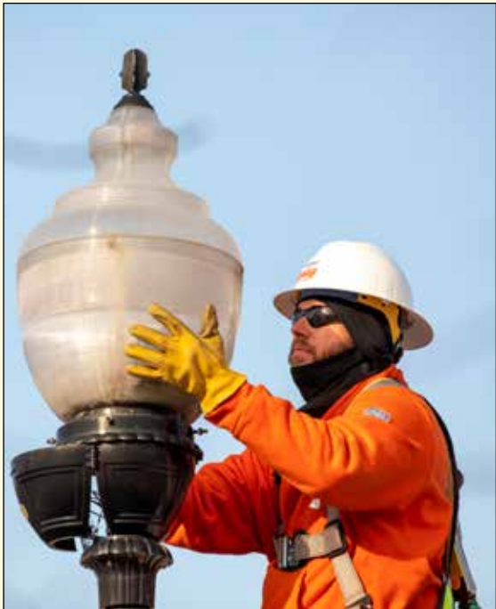
Tim Stambaugh, apprentice streetlight worker, replaces burned out sodium vapor bulbs with new energy-efficient LED bulbs.
